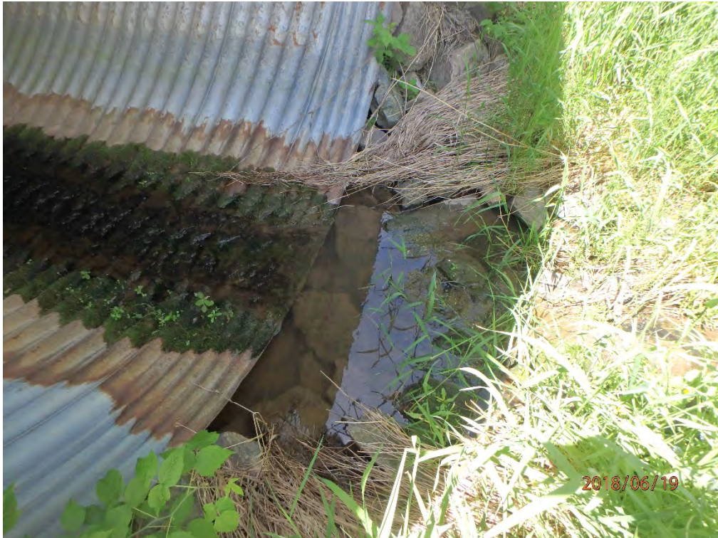
Inlet of culvert, moderate undermining.
