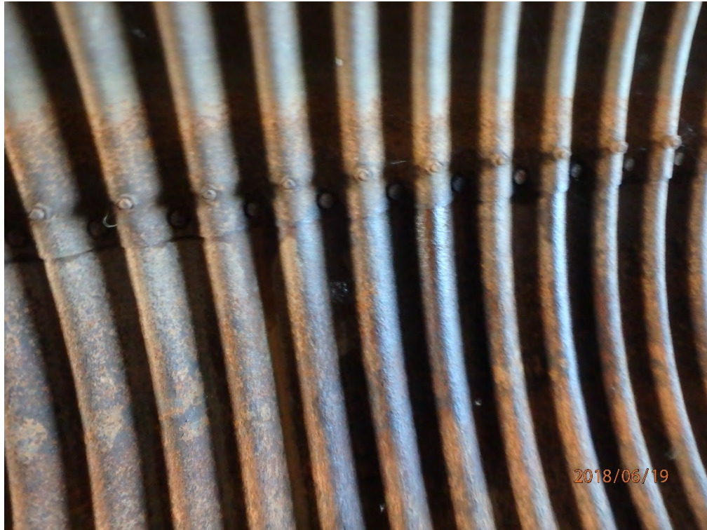
Joint in culvert leaking.
