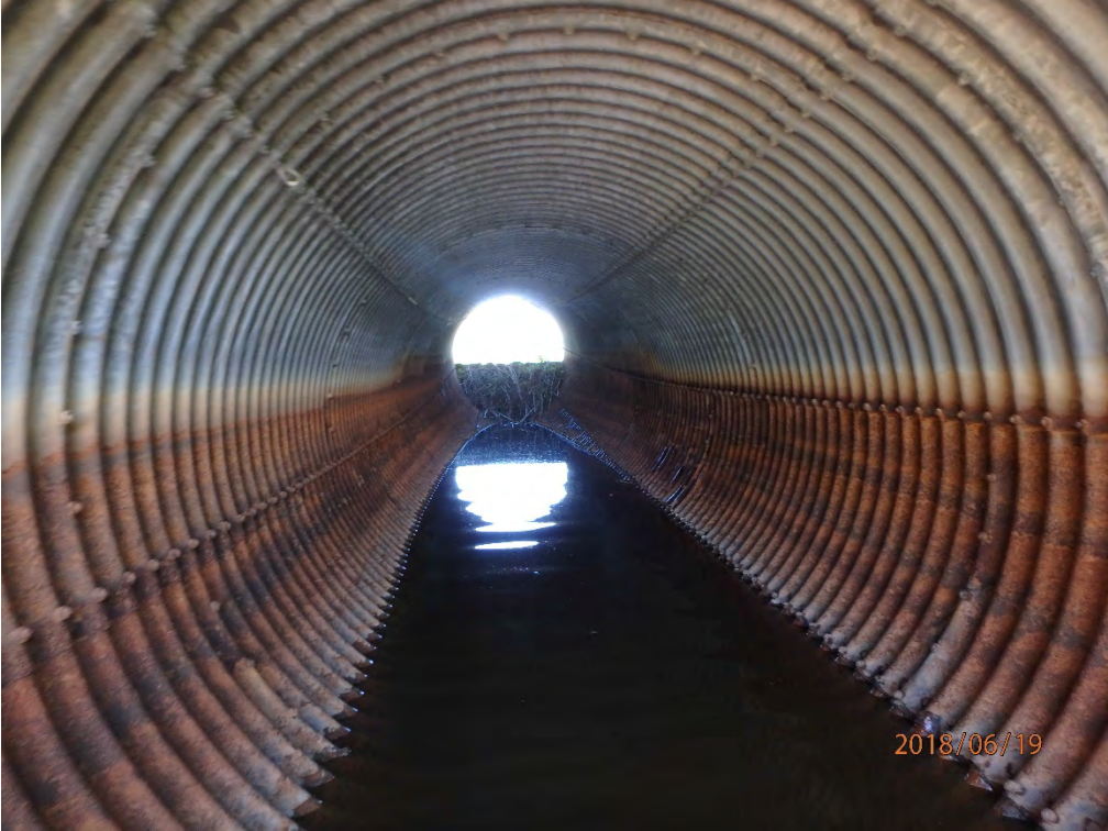
North through the culvert, sag along its length.
