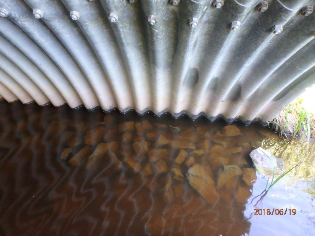
Light staining at waterline
