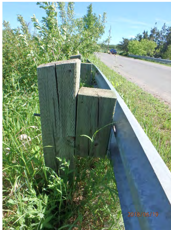
Splits and checks on posts
