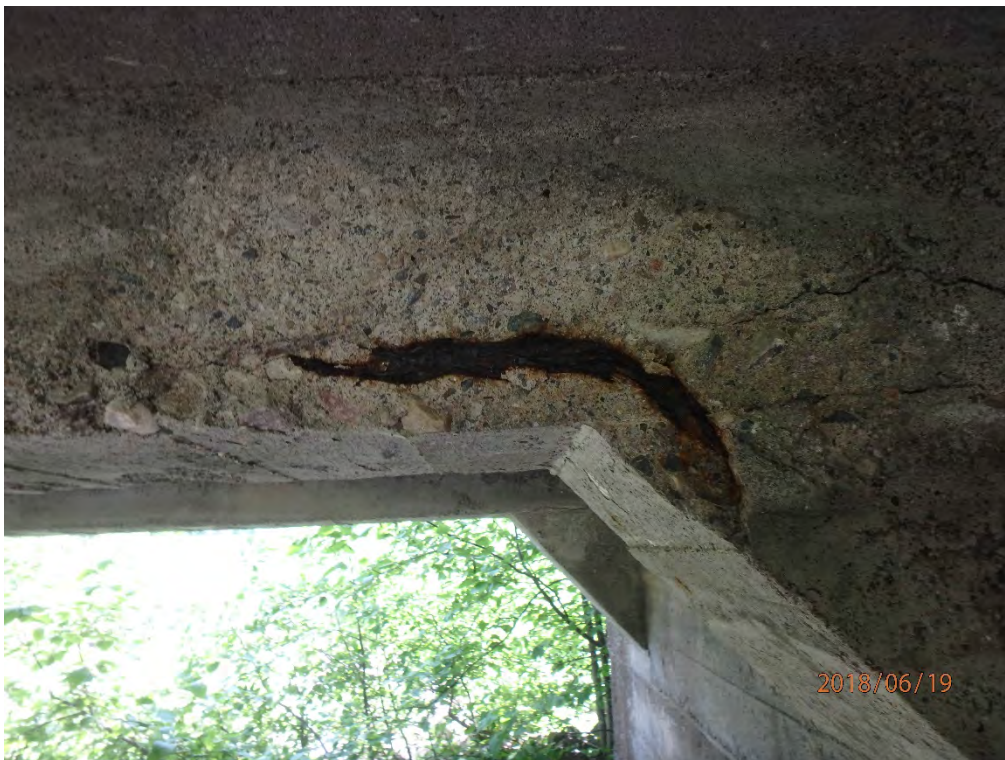
Southeast interior beam with exposed and corroded rebar.
