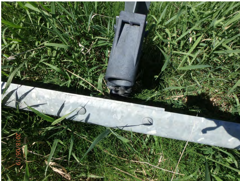
Guidrail support beam missing bolt to connect it to post
