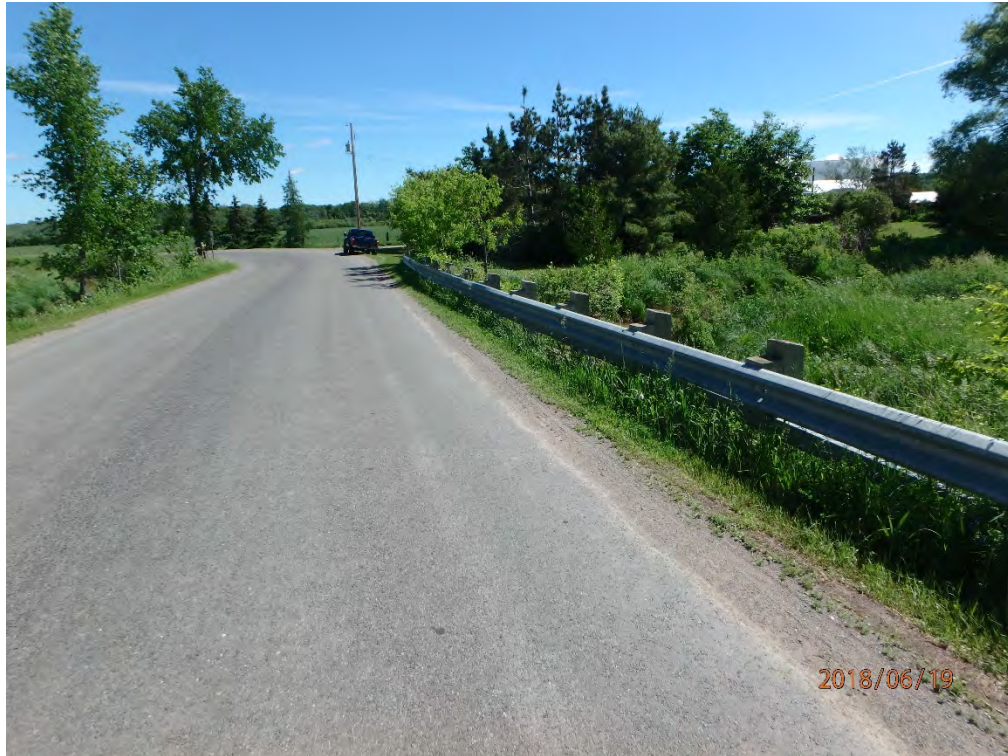
Scraped Guiderail along east side
