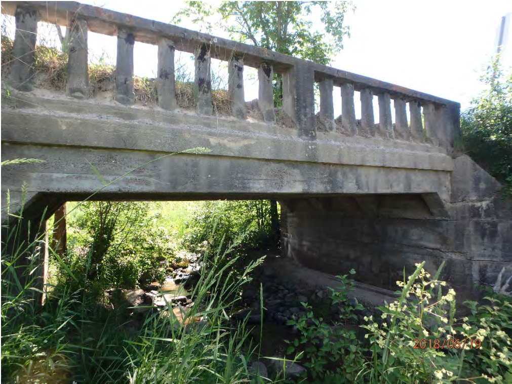
South abutment wall with narrow to wide horizontal cracks, map cracking and delamination.
