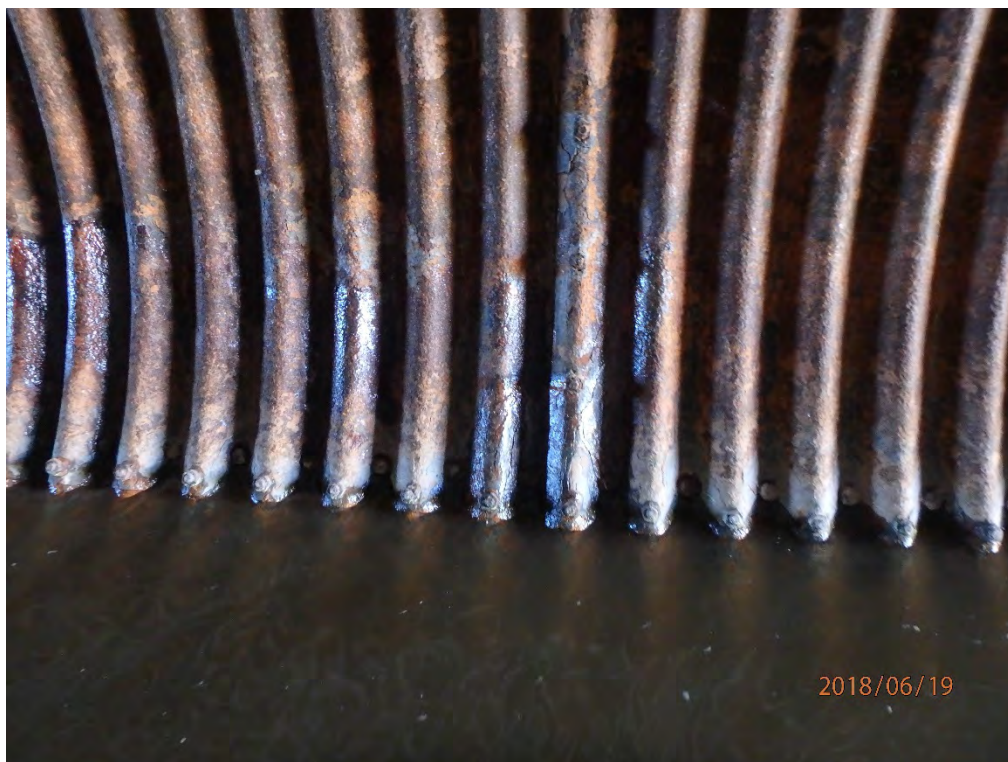
Culvert is rusting and flaking off. Water infiltrating through perforations in metal culvert.
