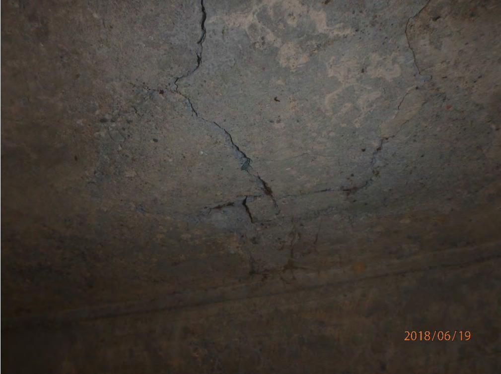
Medium to wide cracking of deck soffit at the east abutment
