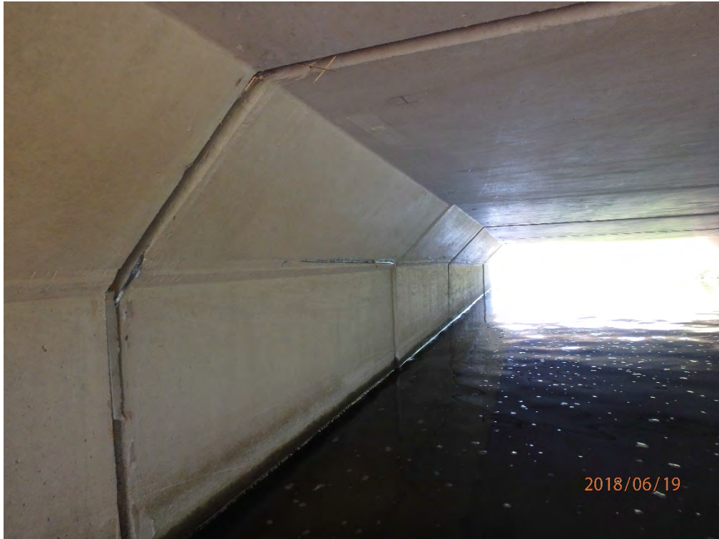
Missing parging at construction joints, typical at all joints.
