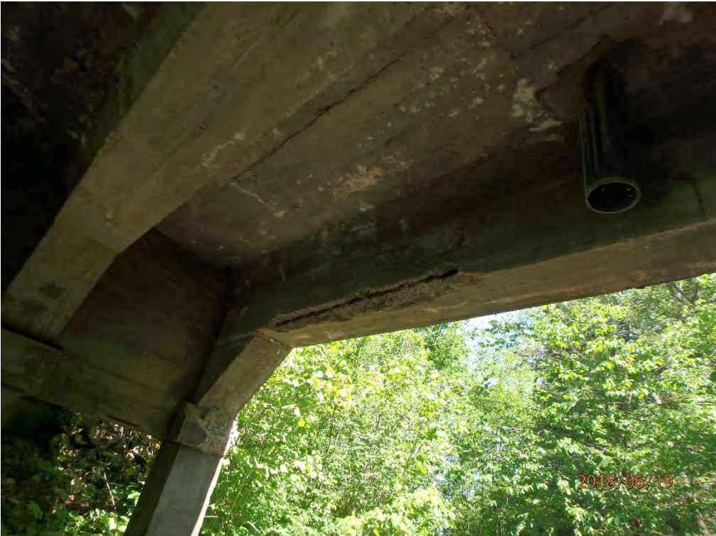
Exposed corroded rebar on east exterior beam.
