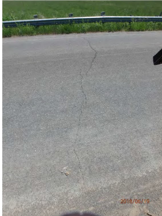
Transverse crack in the wearing surface
