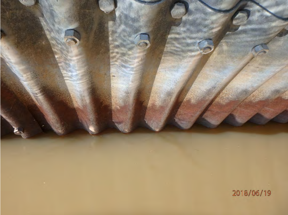
Light to moderate corrosion at waterline
