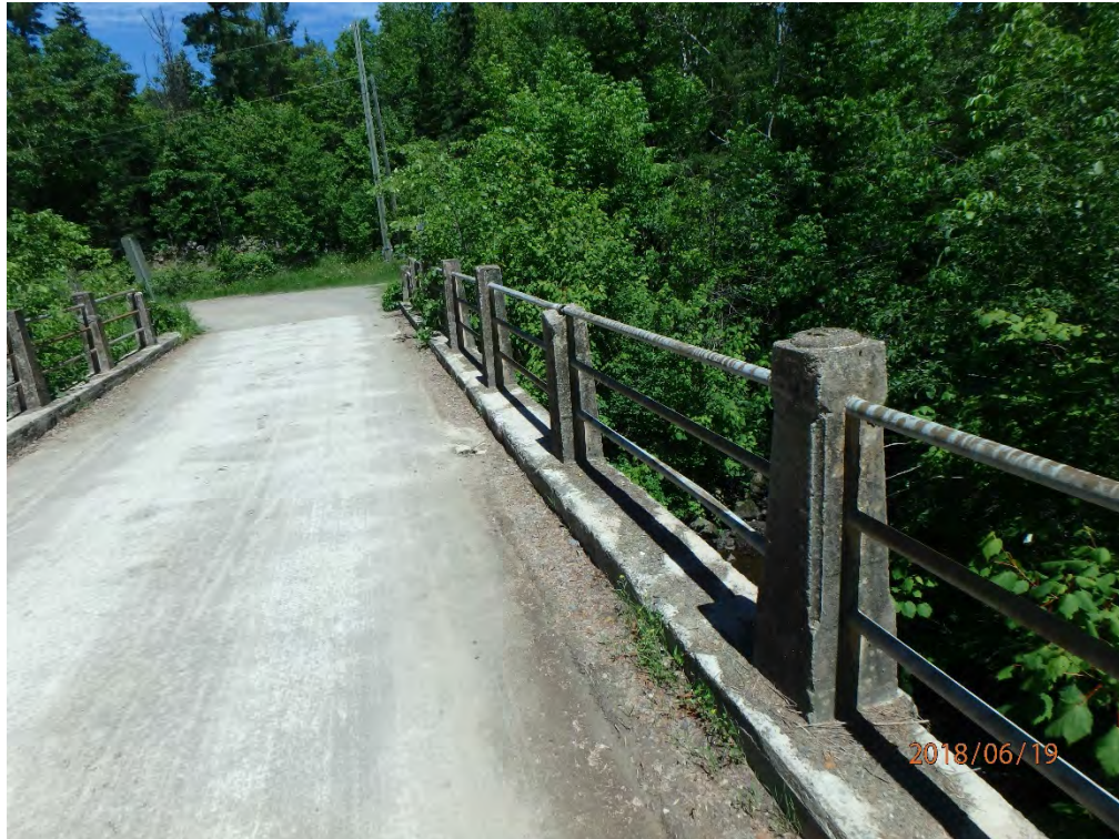
Concrete wear surface with light to moderate scaling. Broken railing post.
