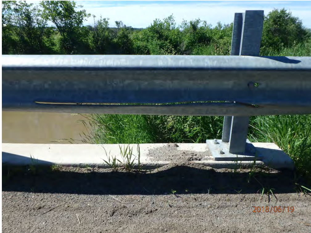
Damaged Guiderail along south side
