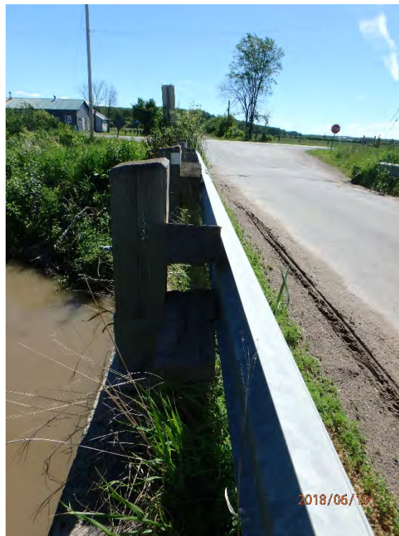
Broken and rotated offset block
