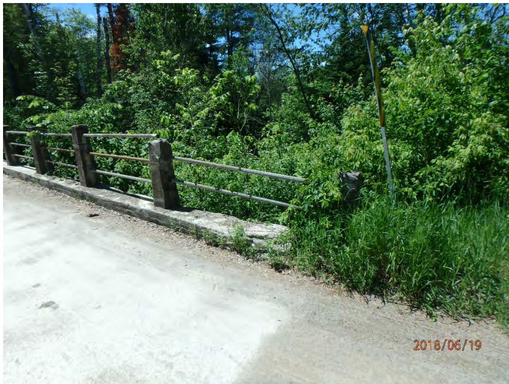
Broken missing railing post. Damaged pipe rails
