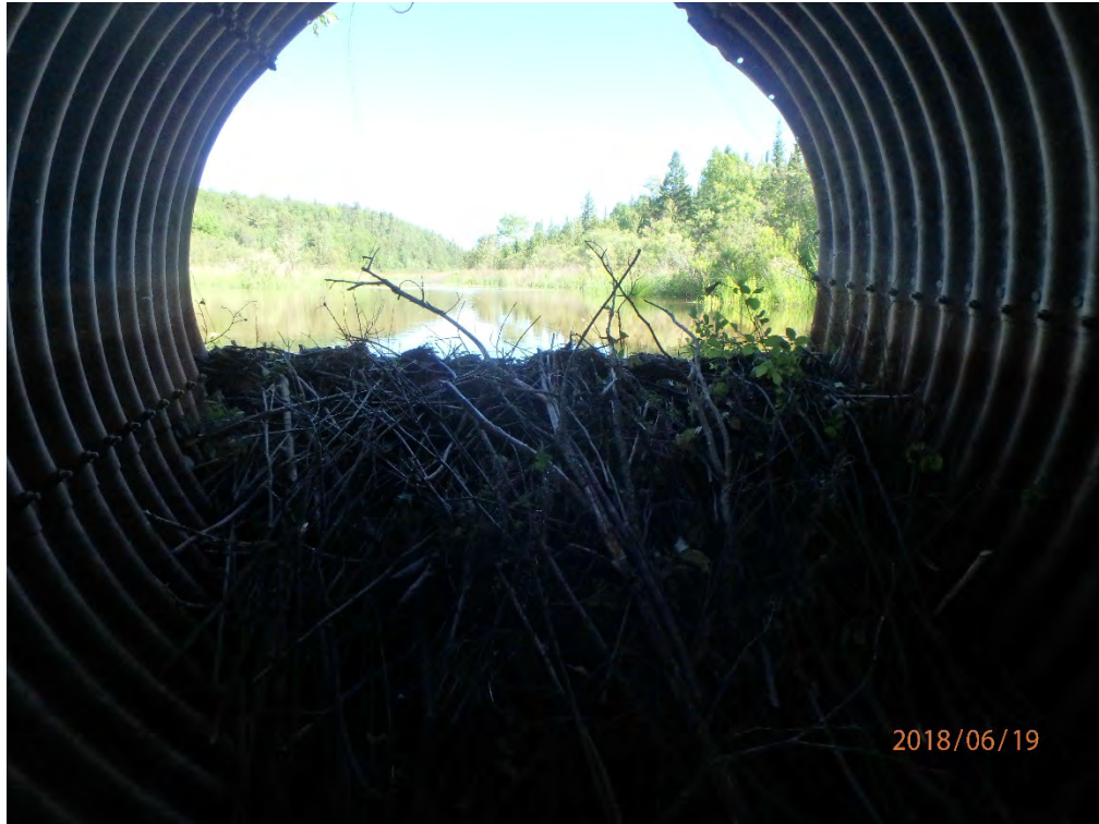
Beaver Dam at the inlet of the culvert
