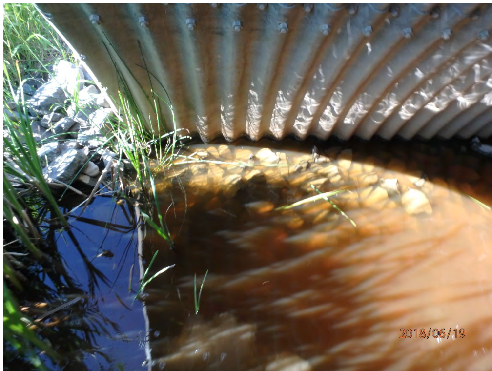
Loss of rock armor at inlet
