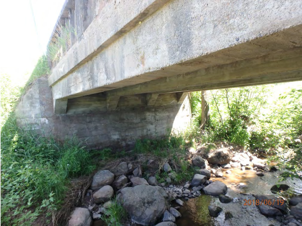
North abutment wall with narrow to wide horizontal cracks, map cracking and delamination.
