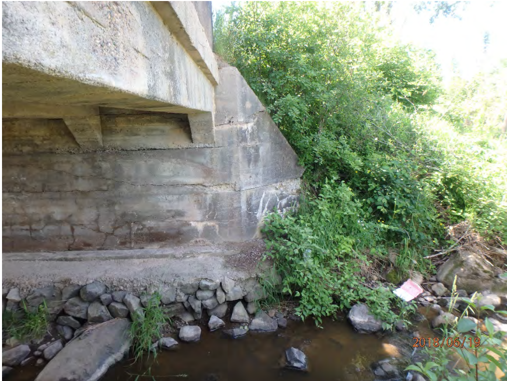
Southeast wingwall with narrow to medium cracking, wide horizontal cracks and delamination
