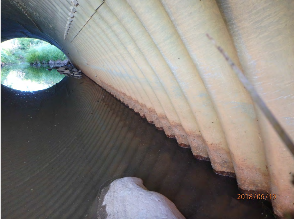
Upstream through the culvert. Minor staining and surface corrosion at just above waterline.
