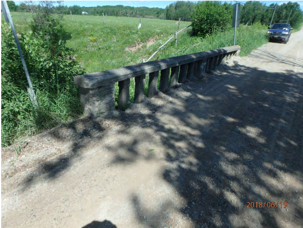
Damage to guard due to impact and buildup of gravel below guard
