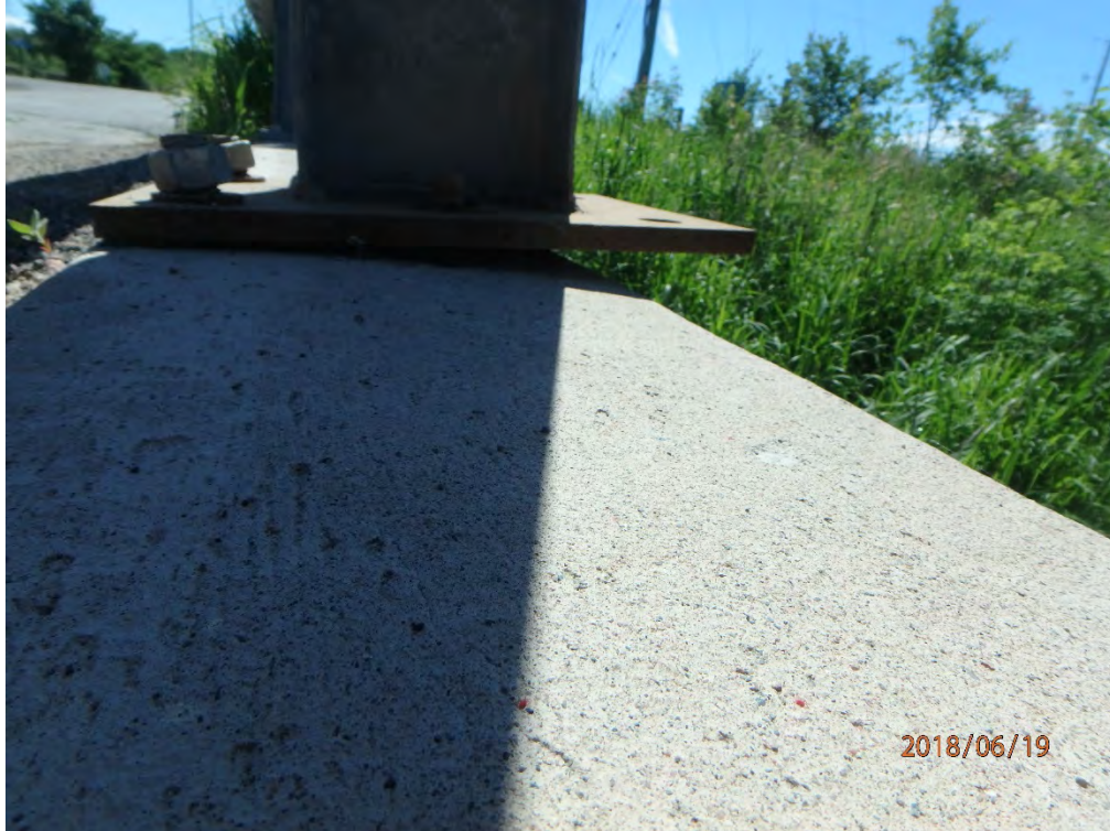
Gap under guiderail baseplate
