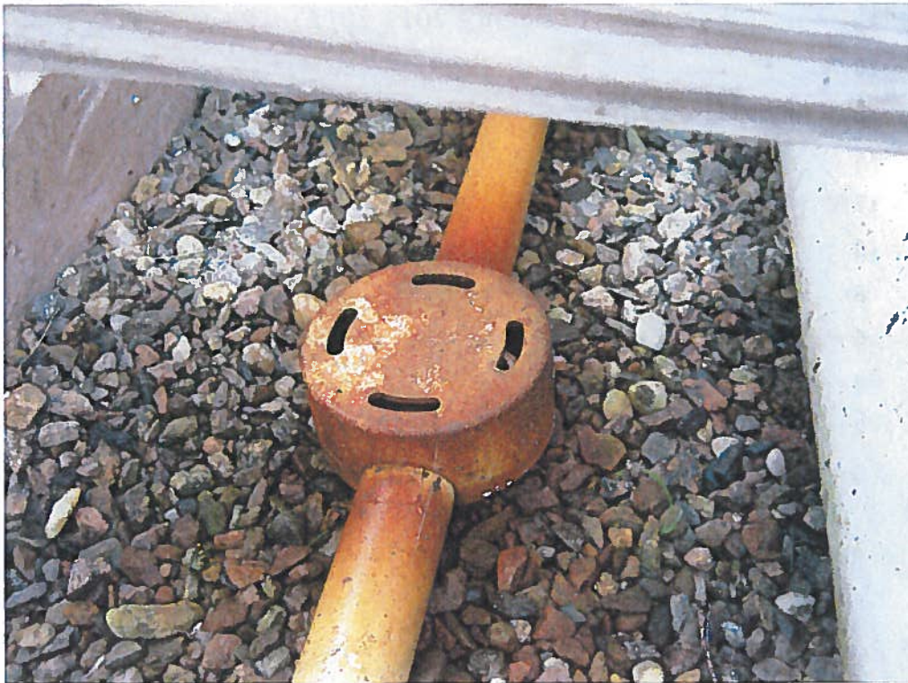
Figure 4. Iron oxide scale coating on distribution pipes and on upper pea gravel in the ETI recirculating sand filter.
