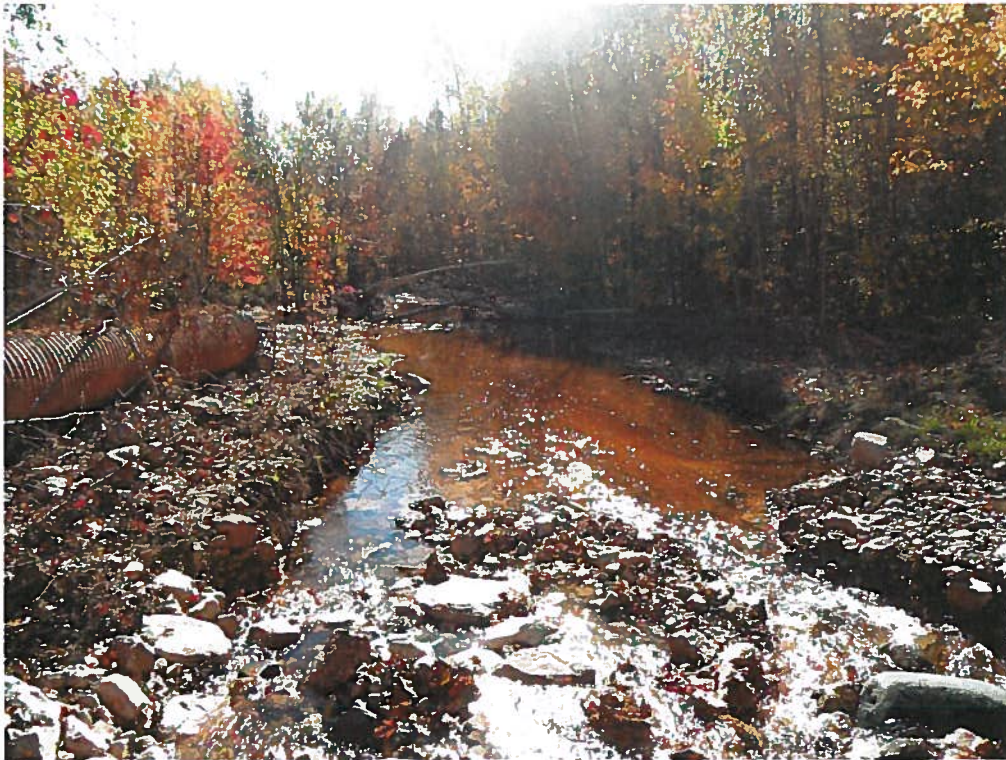
Photographs 19 and 20. Examples of the catastrophic failure of a beaver dam, with bottom photograph showing a road and culvert that were washed out following failure of dam (October 9, 2013).
